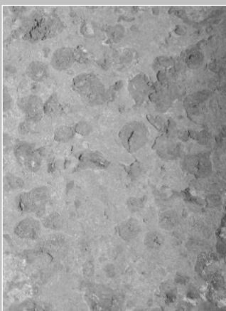
Localised corrosion for high levels of salt
